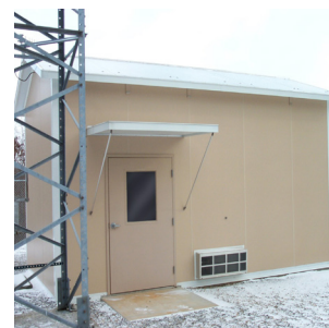
Electric Sub Stations
